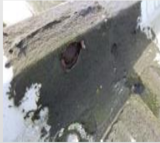
Hole previously repaired with coating
