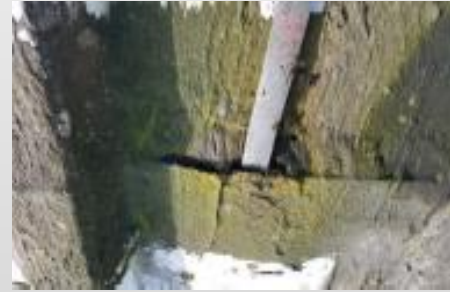
Hole previously repaired with coating
