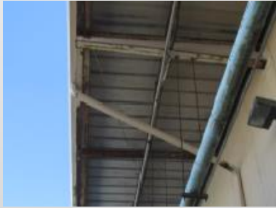
Underside rusted canopy area
